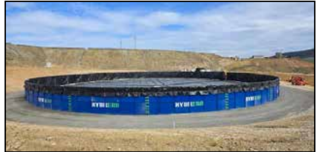
Type of Tank that will be installed in Tank Farm 1
